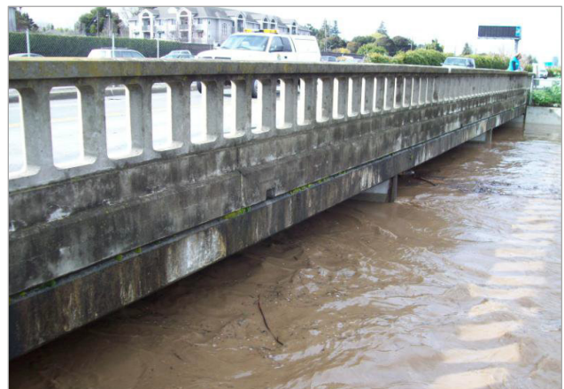
Flooding along San Francisquito Creek.
