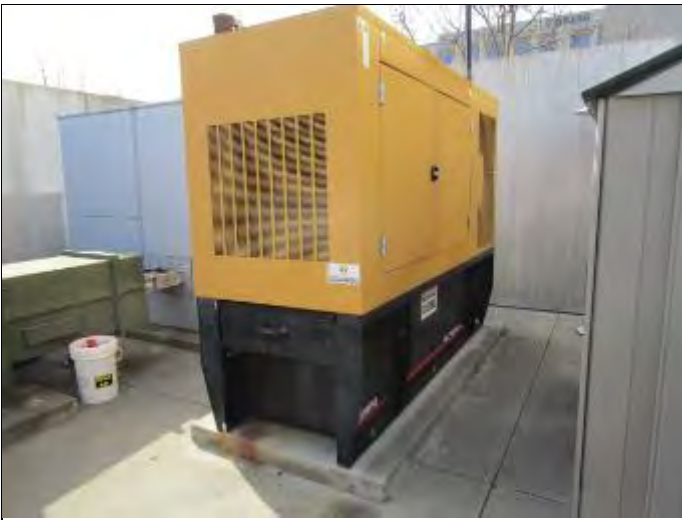
15. Diesel-powered emergency generator in the enclosure south of the 1950 building
