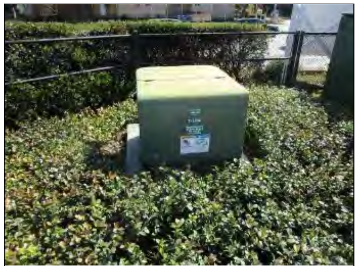
12. Pad-mounted transformer along the southeastern side of the subject property
