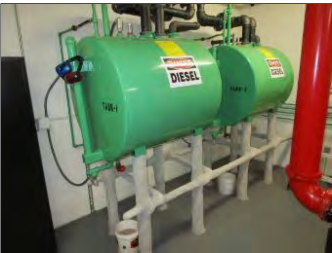
39. Diesel fuel ASTs in the fire pump equipment room
