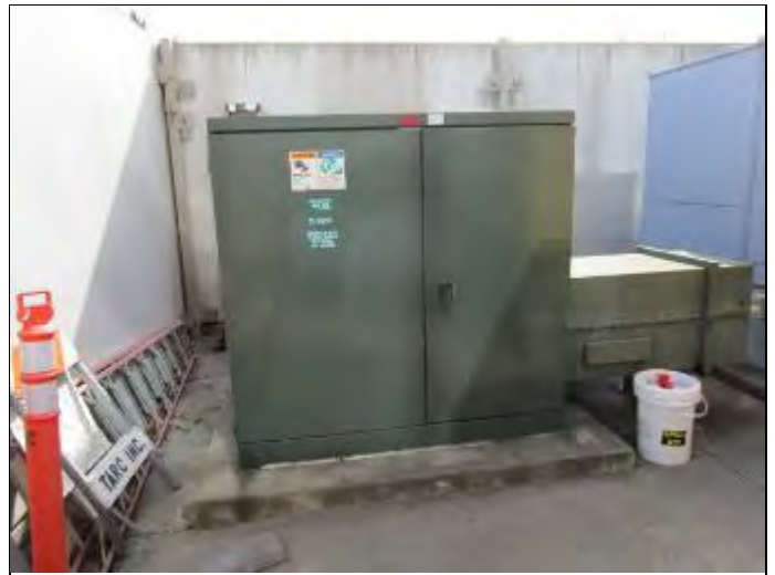
16. Pad-mounted transformer in the enclosure south of the 1950 building
