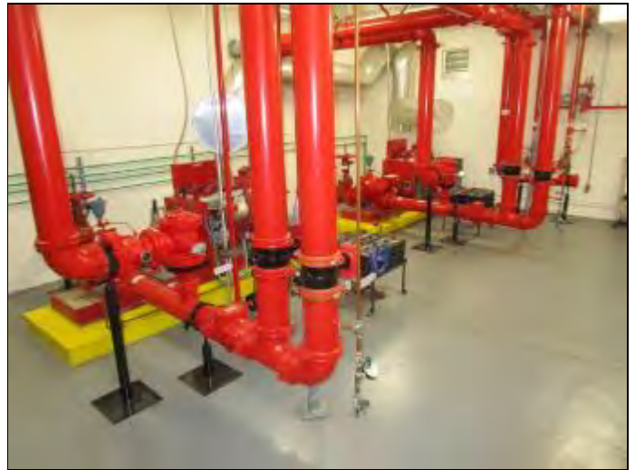
38. Fire pump equipment
