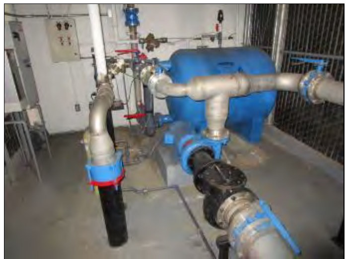
40. Fountain pump equipment
