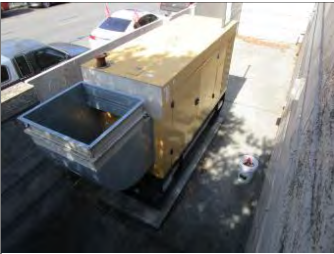
21. Diesel-powered emergency generator in the enclosure west of the 1900 building
