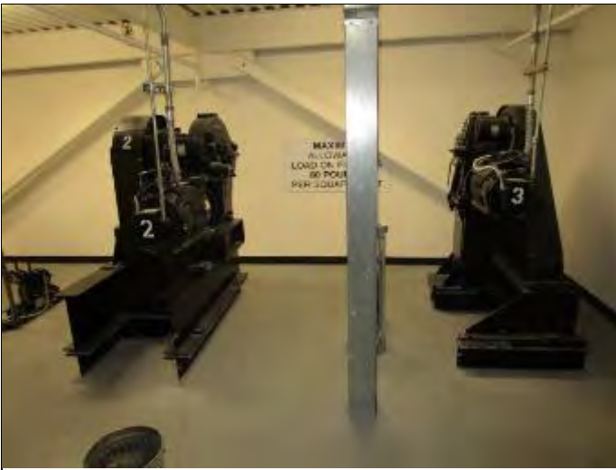
33. Typical overhead traction elevator unit
