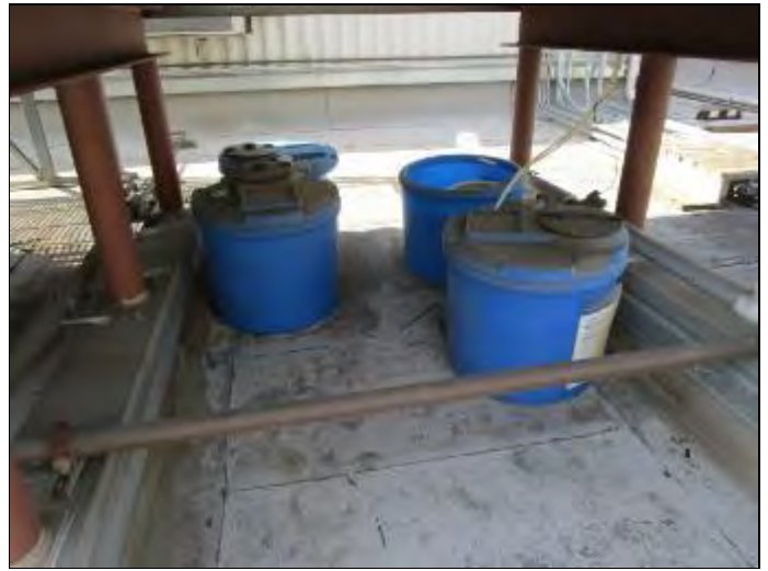
32. Water treatment chemicals on the 1950 building roof
