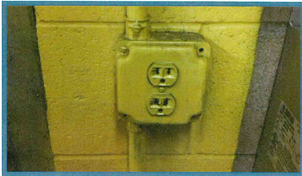
Figure 4-8: Non-Rated Electrical Outlet
