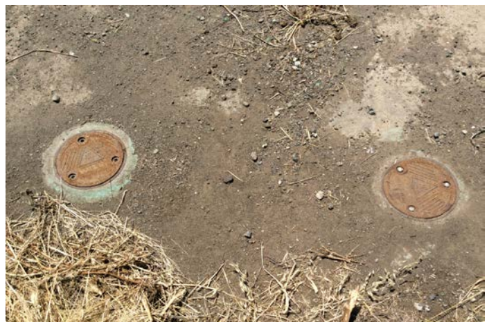
Photo 12: View of monitoring wells on eastern side of site.
